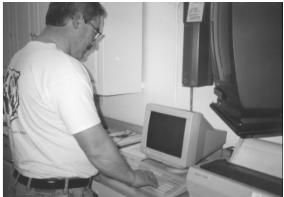
An energy-management system provides real-time information on HVAC operations throughout the building.
