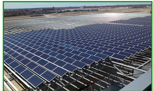
In 2014, the MAC and Ameresco Announce the World's Largest Structure-Mounted Solar Power Installation, Which is Constructed Atop MSP Parking Ramps
