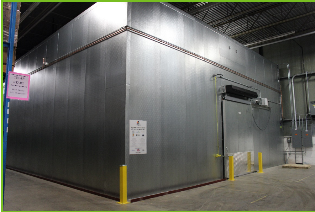
Figure 1. The Food Group, based in New Hope, used a FY2019 GFAP Equipment and Physical Improvement Grant to install a racking system in a new freezer. The increased freezer capacity has made it more possible for their Fare For All program to include locally produced and culturally specific products, such as vegetarian wild rice burgers and locally raised ground beef, in their retail food shares.
