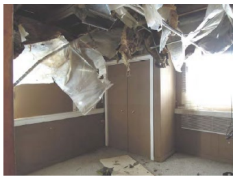
Figure 2: Water damage in living quarters
