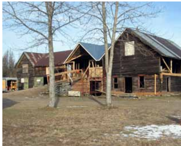
Left: Arson fire, July 2011 (photo courtesy Isanti County Historical Society) Right: Restoration work on the Alex Seitaniemi house barn, December 2012
